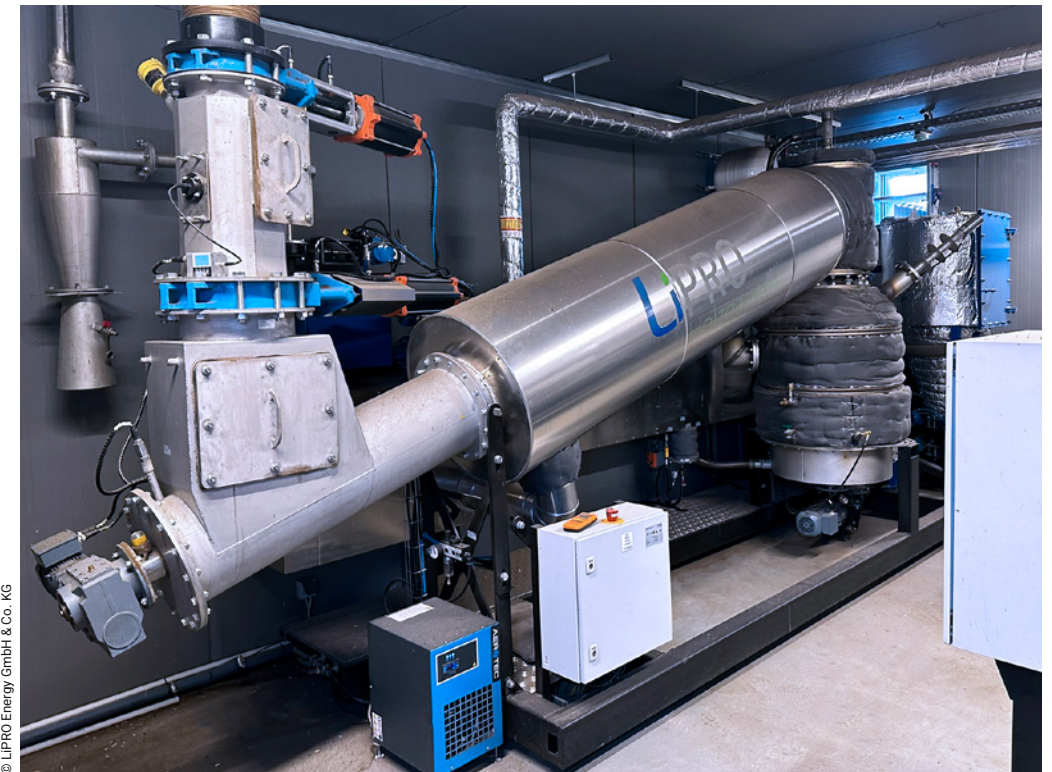
Fig. 41: Wood gas CHP plant operated by project partner LiPRO Energy
