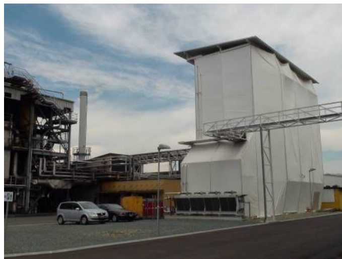
Figure 8: The PDU wrapped in a tarpaulin
