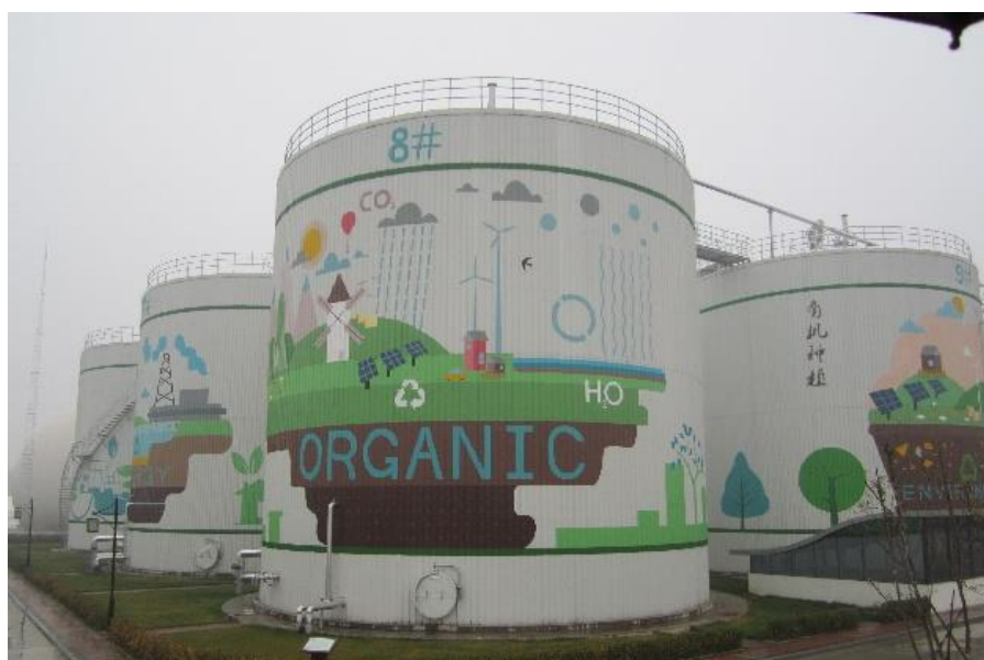
Figure 3: Biogas-Plant in Beijing, China
