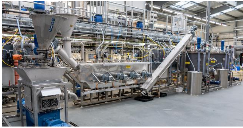
Anaerobic fermentation | Line 2
