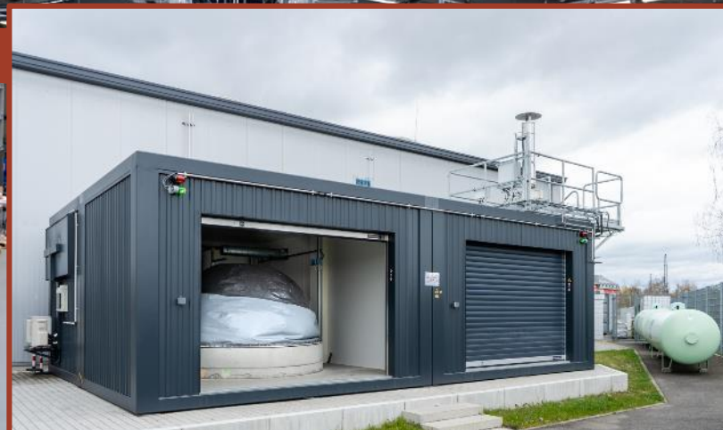
Gas storage & flare
