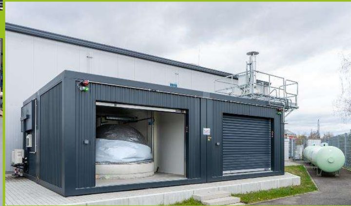
Gas storage & flare
