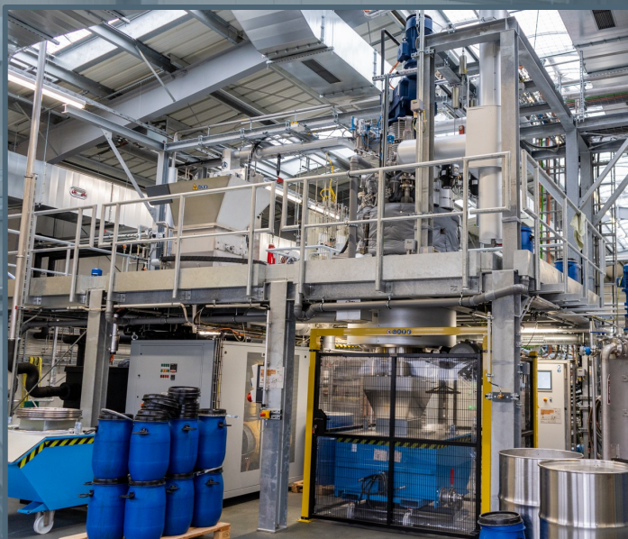
500-L-HT Reactor (Pilot-SBG)
