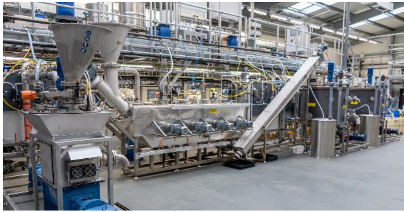
Anaerobic fermentation | Line 2
